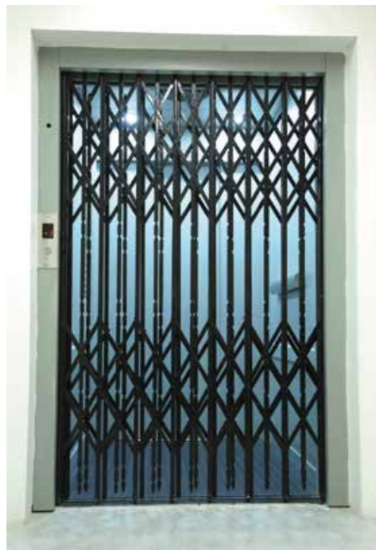
Elevator with Manual Door
