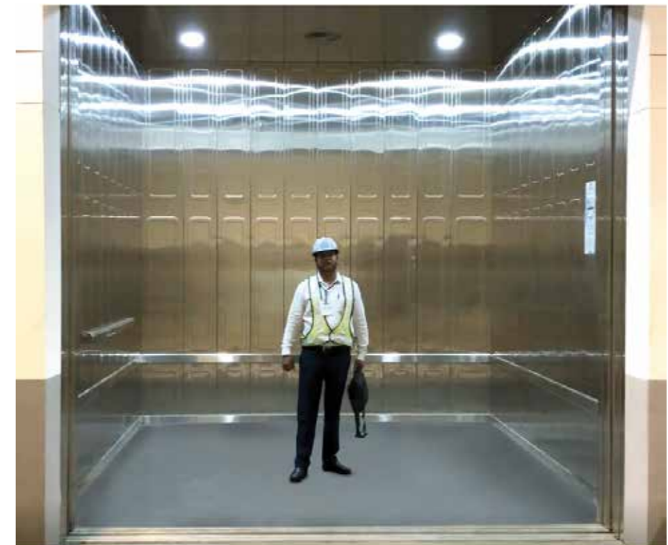
Elevator with Auto & Manual Door
